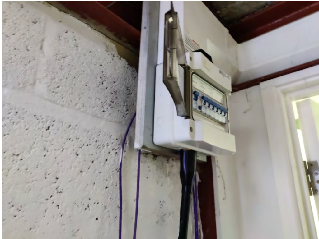
Photo 12: Fusebox at the top of the stairs in the western building.
