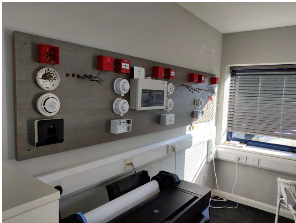
Photo 16: Fire alarms in the eastern building.
