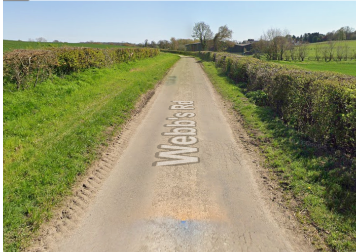
Unclassified road to Streetly Hall Farm, note the verge damage where large vehicles regularly leave the metalled surface. (credit Google)
