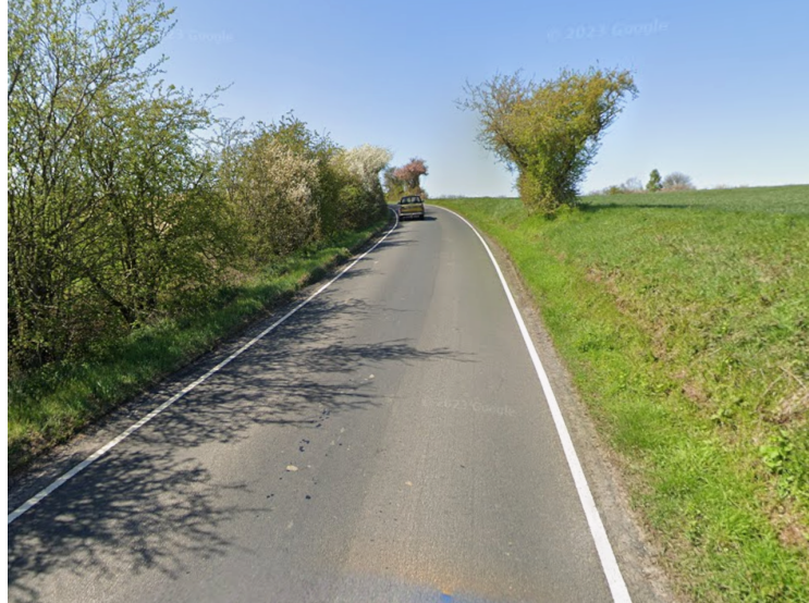
Blind corner & rise on C class road without centre line between West Wickham and Balsham (credit Google)
