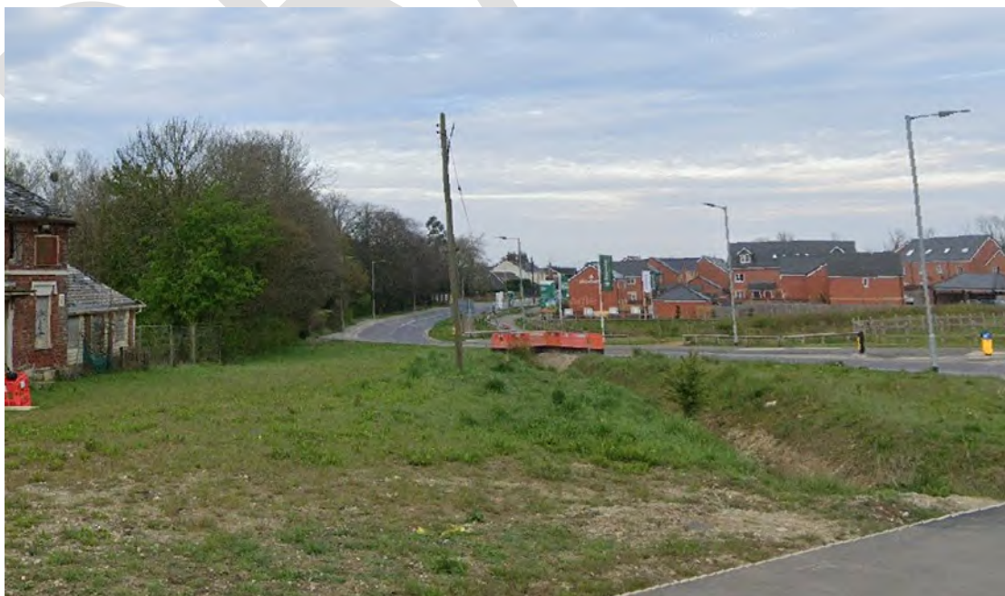
Figure 2.1: Electricity Underground LV and Pole Disconnection
