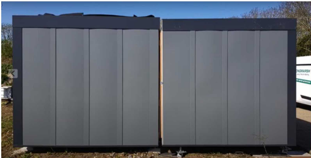
Second half in place just before it is rolled together (see wheels on the feet) and joined.
