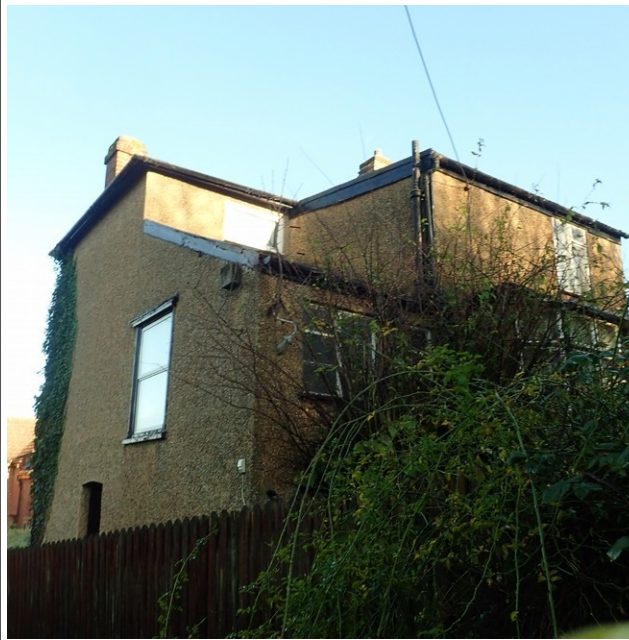
Figure 6: View of western aspect from lane, showing rear "roof box" with flat roof
