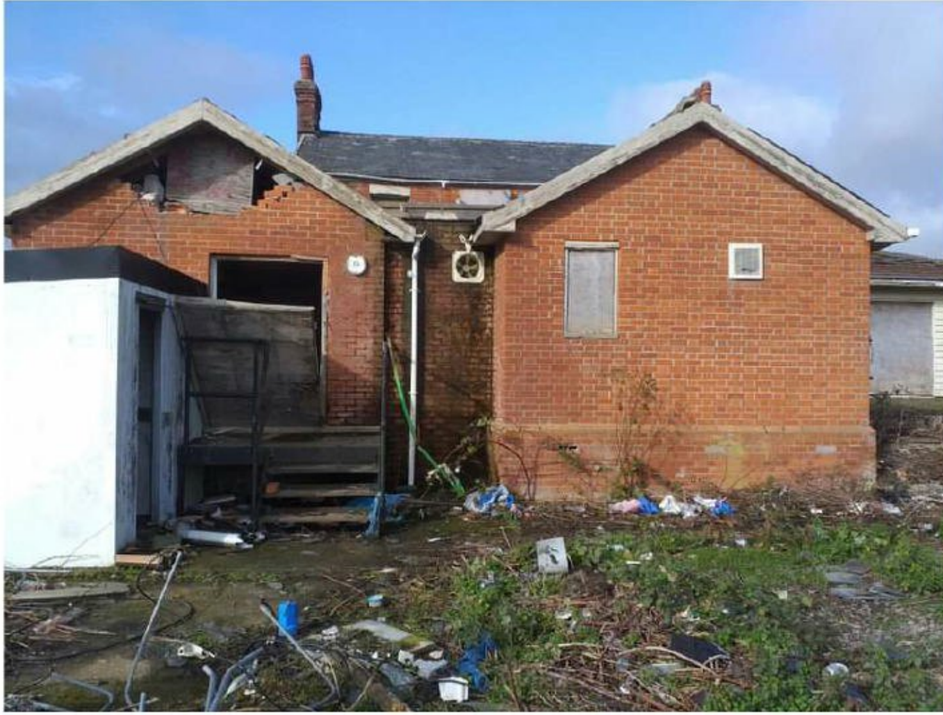
Hole in wall in south eastern section of building
