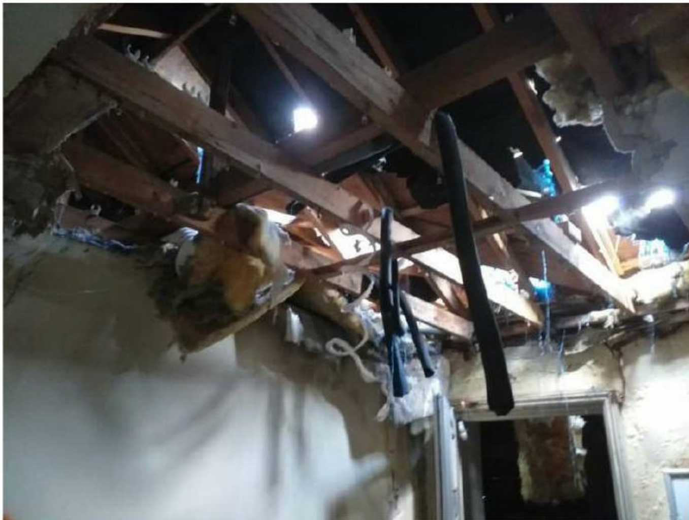
Damaged section of roof in eastern section of building
