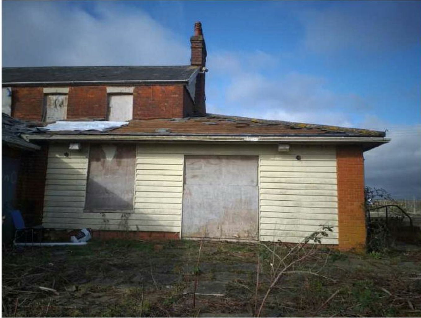
North eastern elevation. Missing roof tiles
