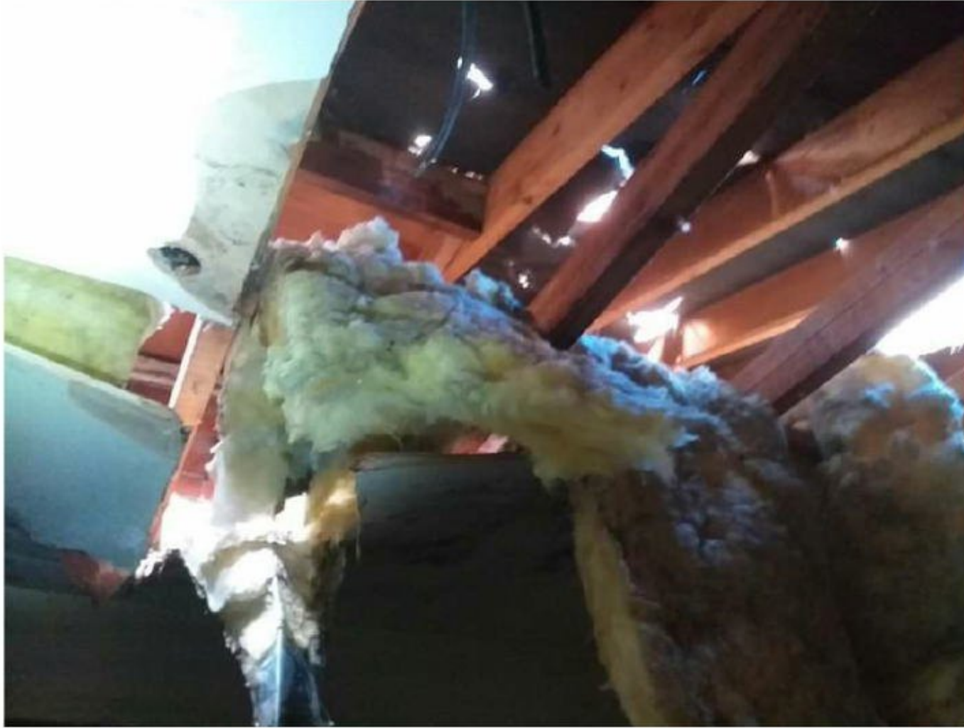
Damaged section of roof in north eastern section of building & hole in roof
