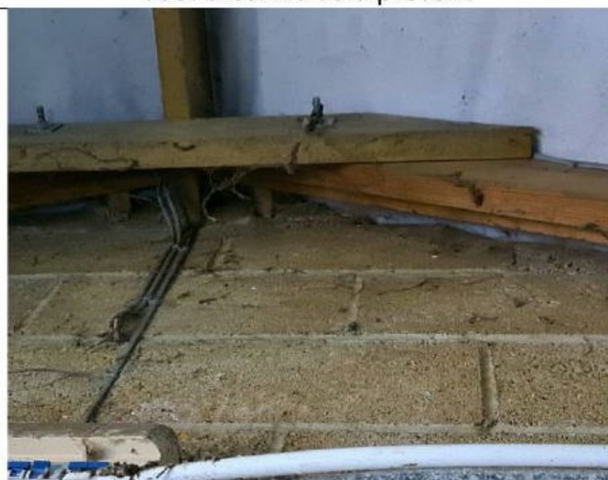
Structure 1- Gap between blocks and roof felt at gable end of stable block
