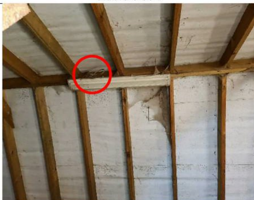
Structure 1- Lighting in stable block with swallow nest present (TN1, circled red)
