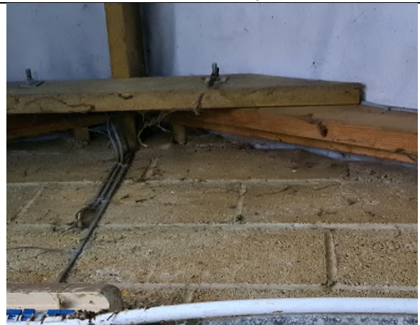
Structure 1- Gap between blocks and roof felt at gable end of stable block
