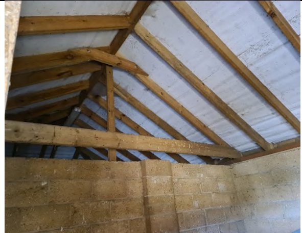
Structure 1- Internal of stable block with breathable roofing membrane visible under roof tiles. No void present
