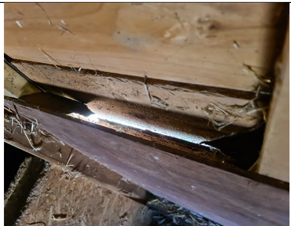
Structure 2- Eastern side internal, gaps present in timber cladding
