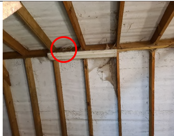
Structure 1- Lighting in stable block with swallow nest present (TN1, circled red)
