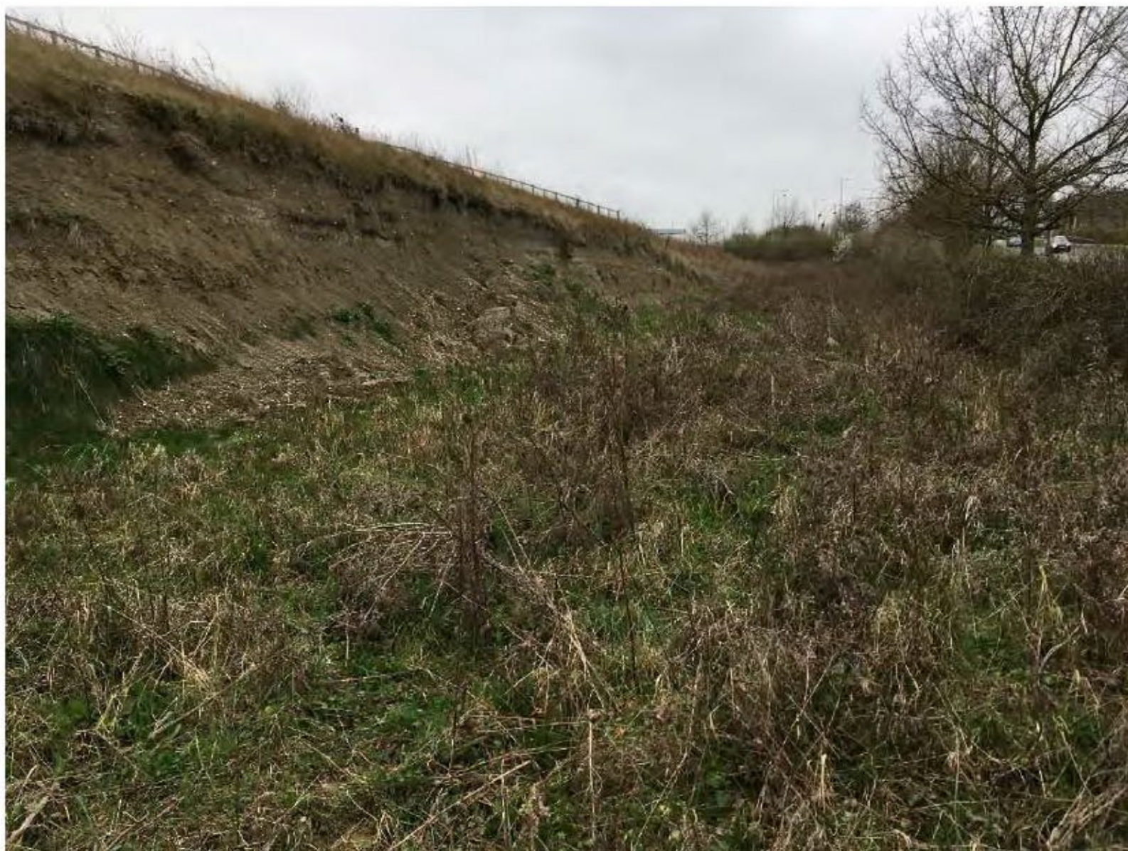
Photograph 6 – Earth bank created by slope failure
