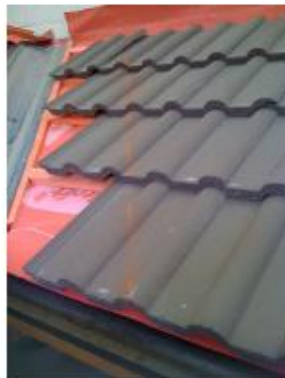
Line struck - two tile widths from desired finishing point in valley line
