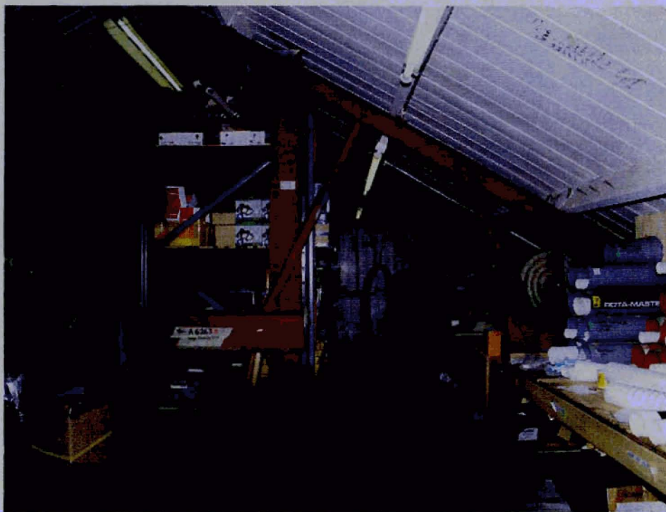
Plate 18 Roof and cut away steel frame to accommodate first floor in Building 8
