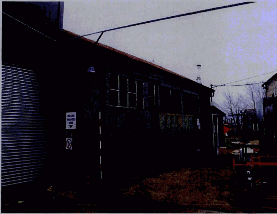
Plate 17 Exterior south east elevation of Building 8 and rear extension of Building 3 taken from SE
