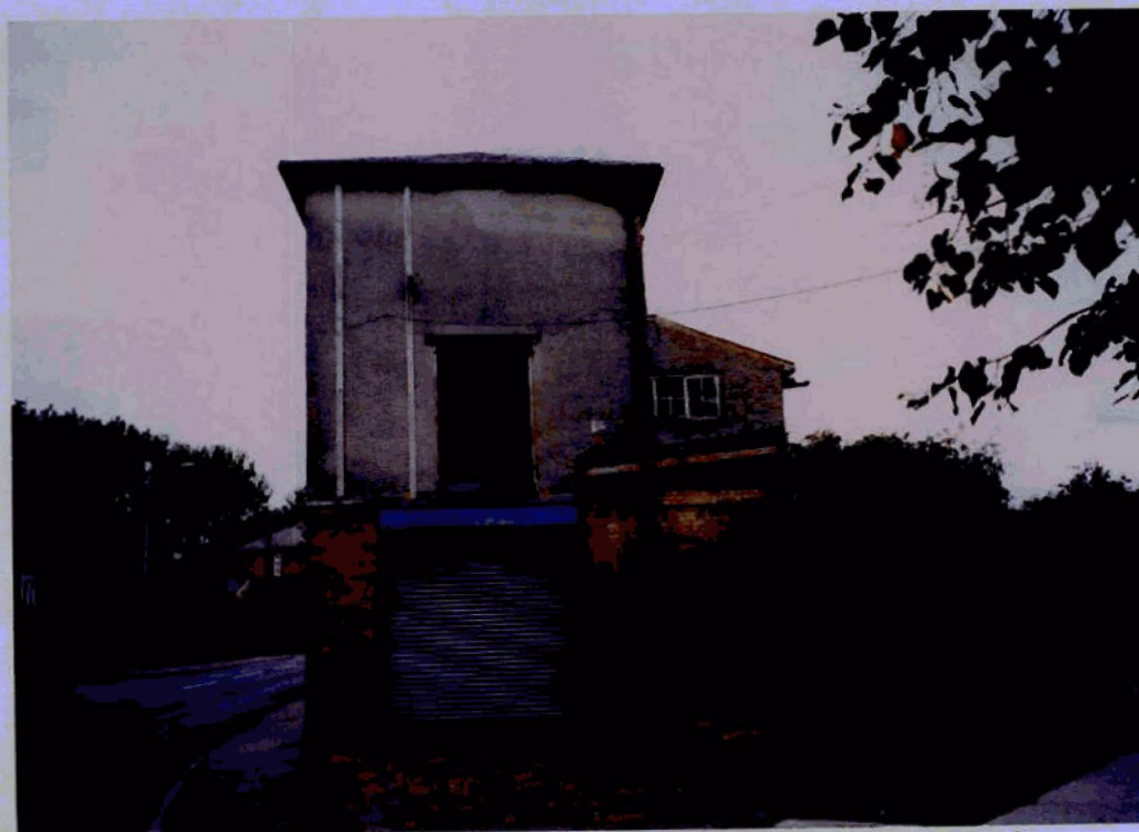
16. Detail of East gable of Silk Mill - Rear extensions to be removed
