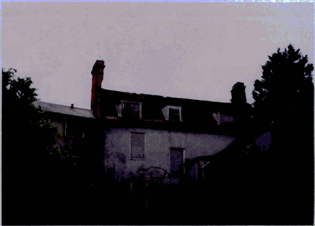
21. Existing rear façade of Hamlet House and abutment to the Silk Mill.
