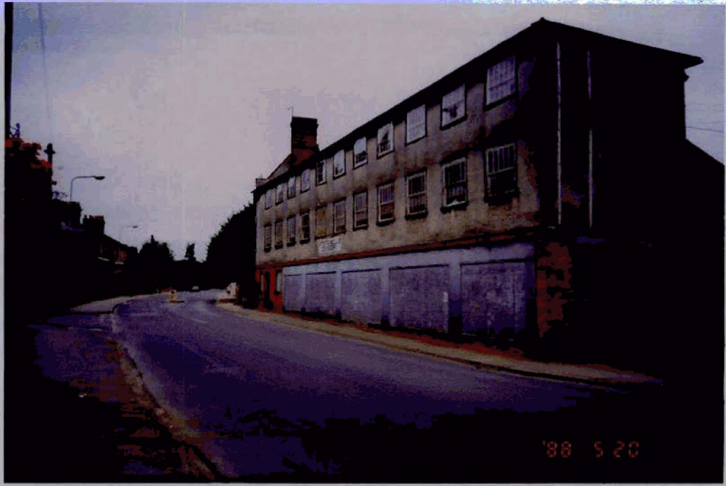
13. Looking West along Hamlet Road – full extent of existing Silk Mill façade showing blocked-up openings at ground floor level.
