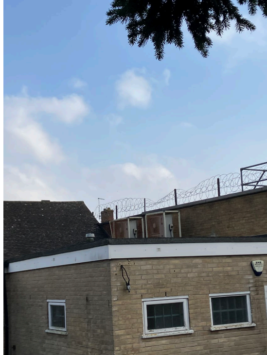
Figure 4 Existing 2no AC condenser units
