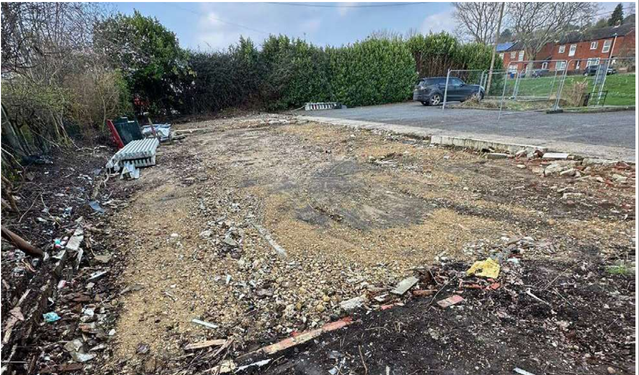
Photo 4: View of the southern portion of the Site where the previous office unit was removed.
