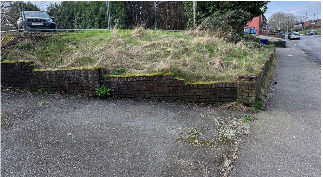
Photo 2: Grassed embankment with a small retaining wall along the access driveway in north of the Site.
