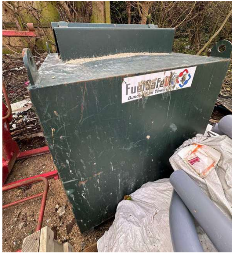
Photo 5: Currently empty (at time of walkover) 500L white diesel tank.
