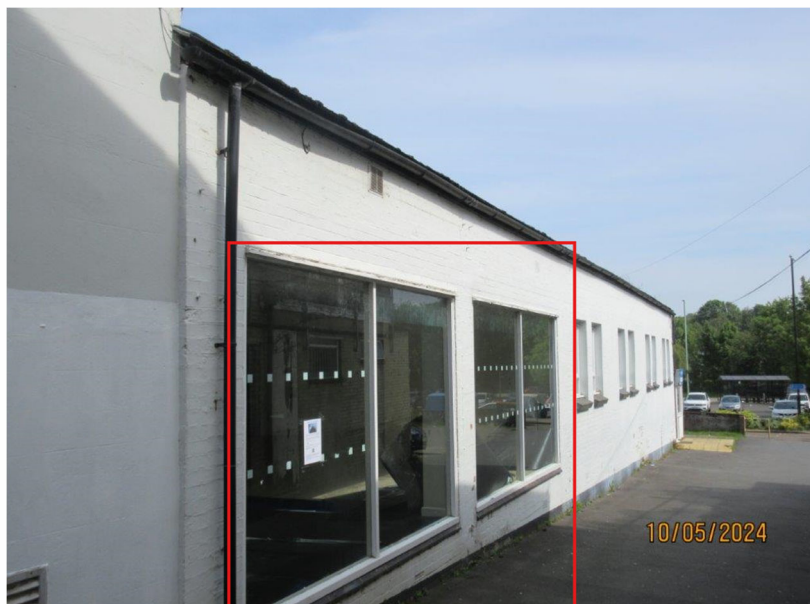
Photo 1: Side elevation with windows highlighted that are to be reduced in size
