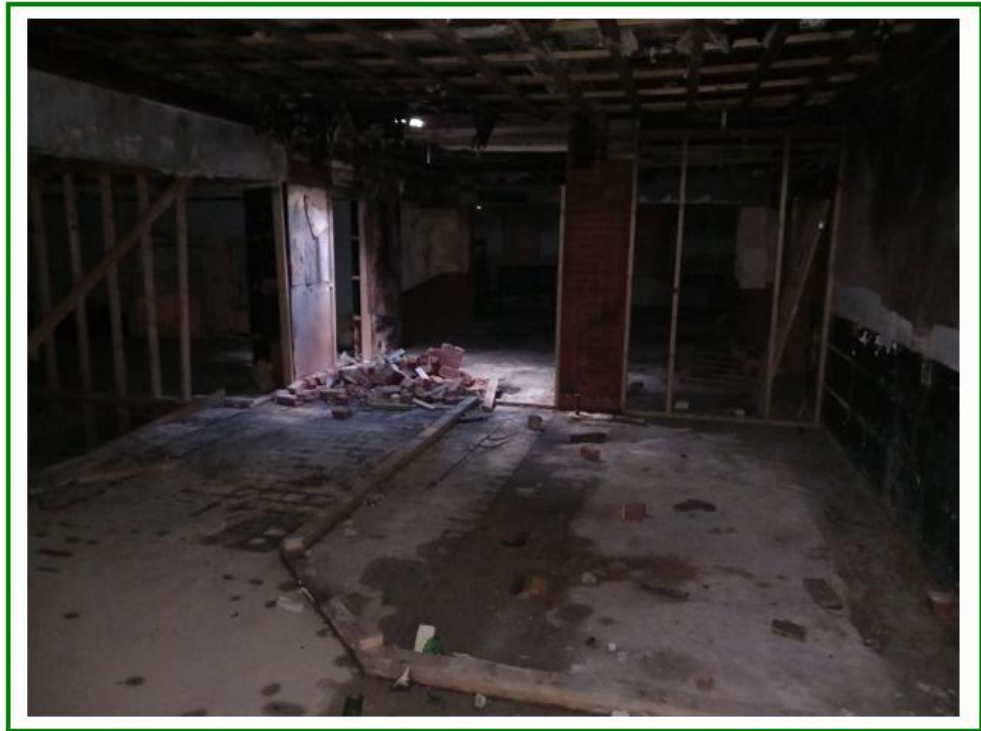
Photo No.16: Further shot of the interior showing the dilapidated, stripped nature of the interior of the onsite structure
