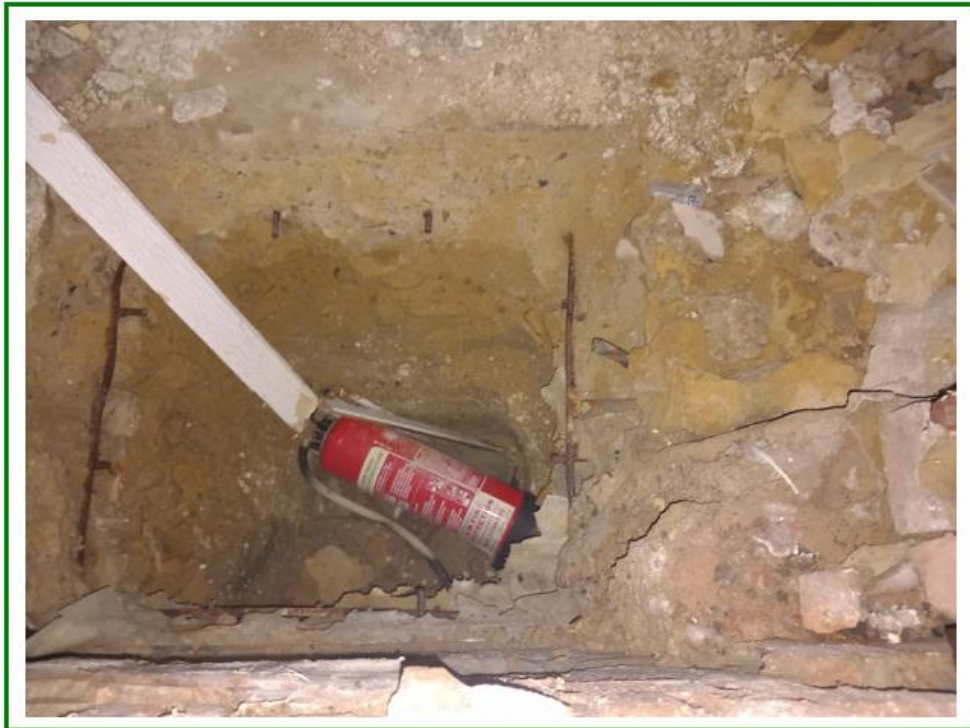
Photo No.18: Second inspection pit noted within the structure showing limited made ground deposits atop gravelly sands
