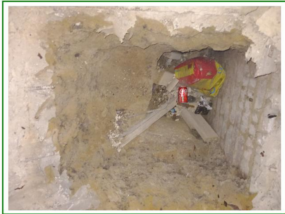
Photo No.20: Third inspection pit noted within the structure showing limited made ground deposits atop gravelly sands
