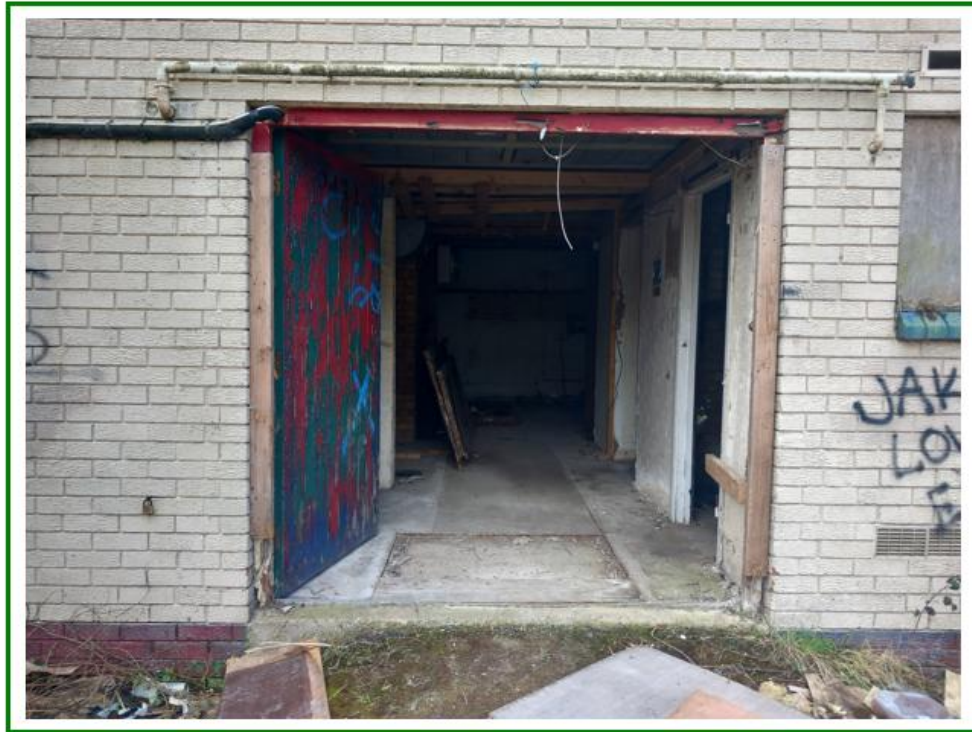
Photo No.14: Facing SW outside the NE face of the building showing access to interior
