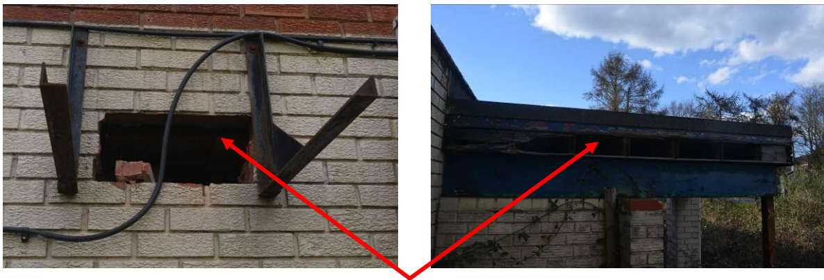
Figs. 5 & 6 External gaps and potential access points (arrowed)
