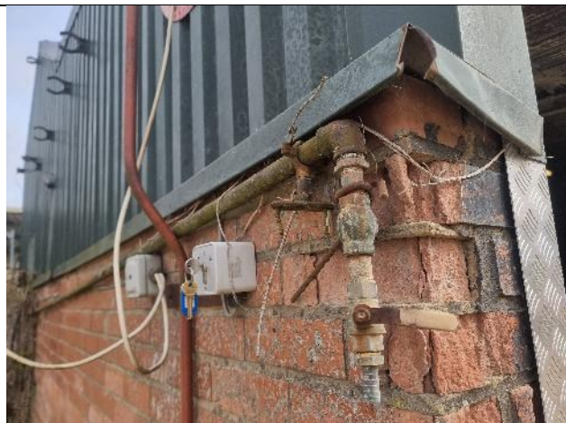
Photo 11: Cracks in brickwork of B1.
