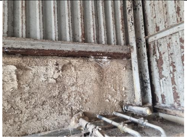
Photo 14: Gap internally in B1.
