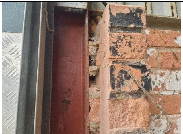
Photo 12: Gaps in brickwork inside of B1.
