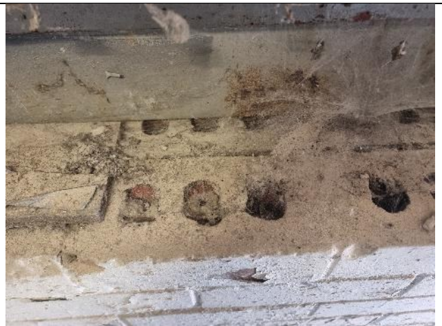
Photo 16: Gaps in bricks in B1.
