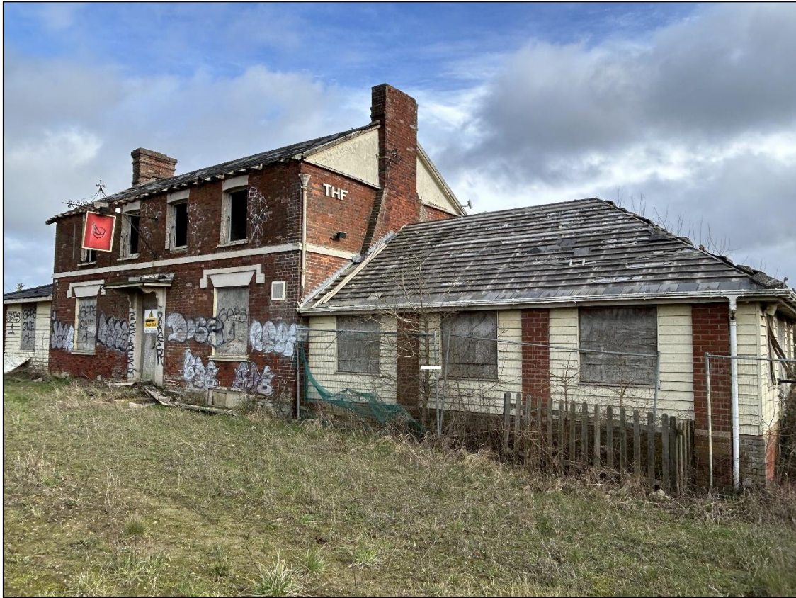
Plate 1 – Western elevation of the Fox Public House, note poor condition
